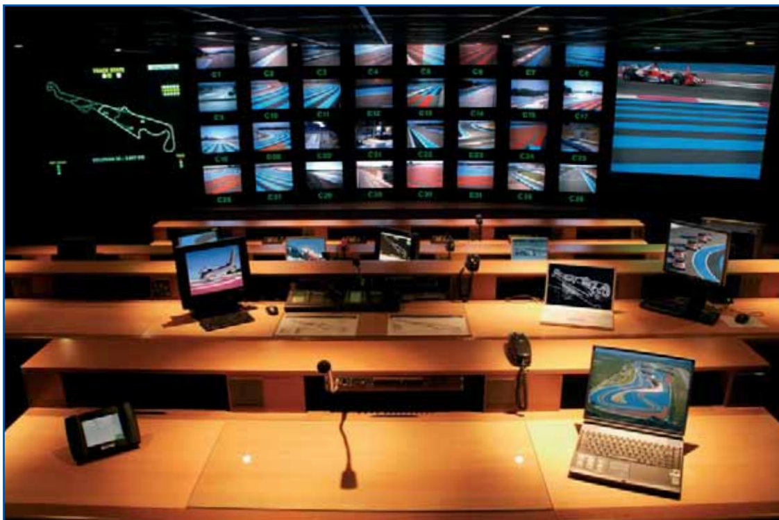
CPR 8- Track Video Control Room
